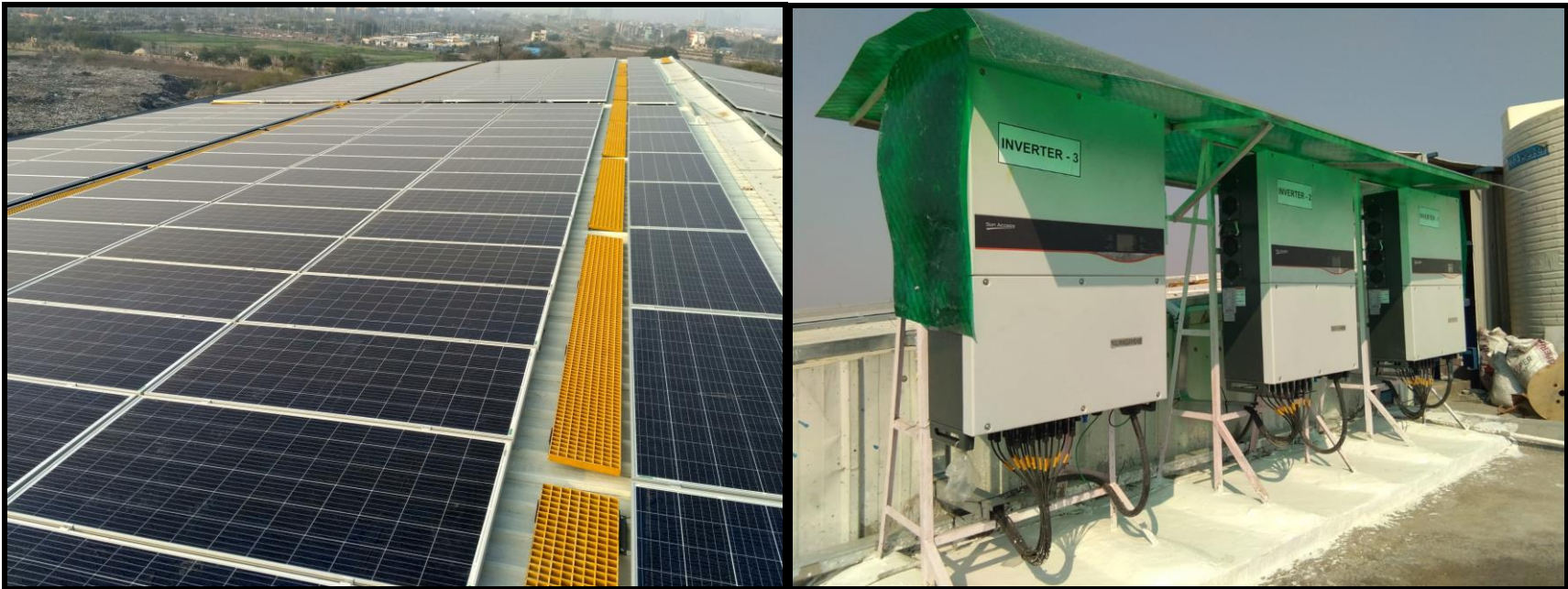
United Exim, Noida (UP) 225kWp rooftop SPV installation
